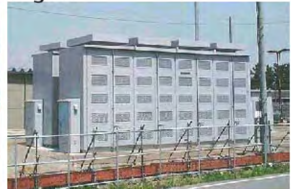
Sodium Sulfur (NAS) Battery
